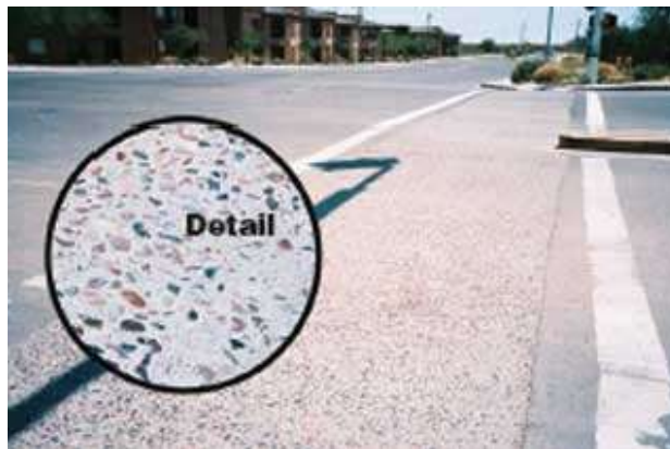
Figure 6-2—Some agencies use concrete surfaces with a water wash finish to improve horse traction. This treatment may not be suitable in all areas.
