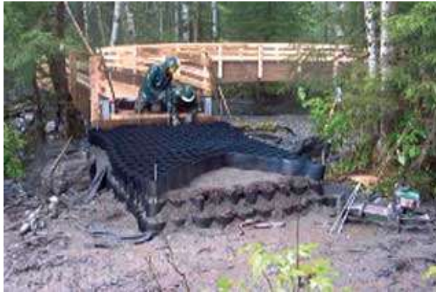
Figure 6-4—Workers are preparing the third layer of geocells at a trail bridge approach. The cells provide structure for soil that forms the tread.
