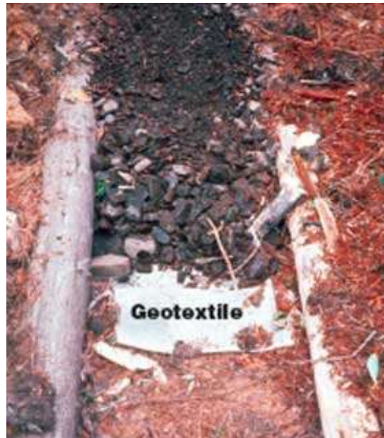
Figure 6-3—Geotextile is sandwiched between a substandard soil base and an aggregate cap to prevent soil migration. Logs hold the edges of the fabric in place.
