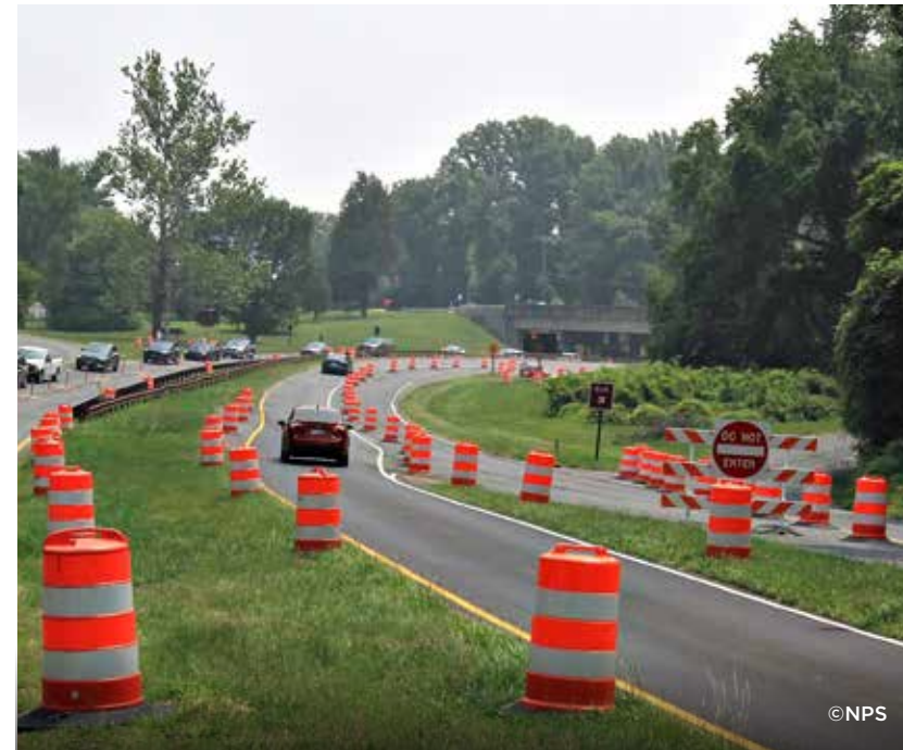
Project to reconstruct 7.6 miles of the George Washington Memorial Parkway in Virginia . The project is critical to improving the driving experience, safety, water drainage and the scenic views on the parkway. The George Washington Memorial Parkway is a commuter road that roughly 70,000 vehicles drive on daily.
